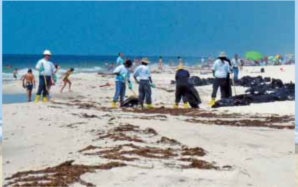
The hand crews work during the day below the tide line where it's wet, while the BeachTech's work all night, giving BP the best cleaning efficiency.
